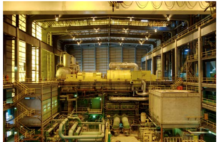
Inside Tarong Power Station's Turbine Hall
