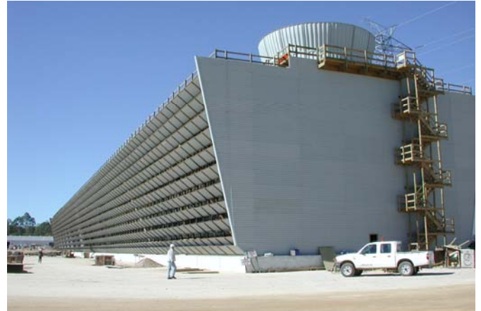
Tarong North's Cooling Towers
