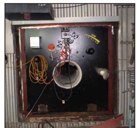
Progressive installation of low NO x burners in Unit 2
